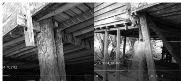
Fig 1. The pillars of the damaged traditional house building supported by wooden supports.
